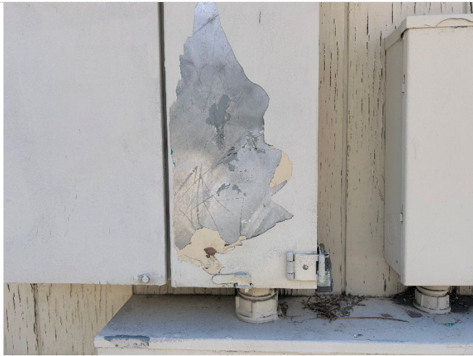
Cream Paint on Metal Electrical Box
