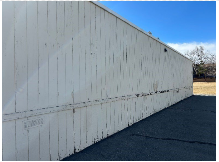
Cream Paint on Wood Siding
