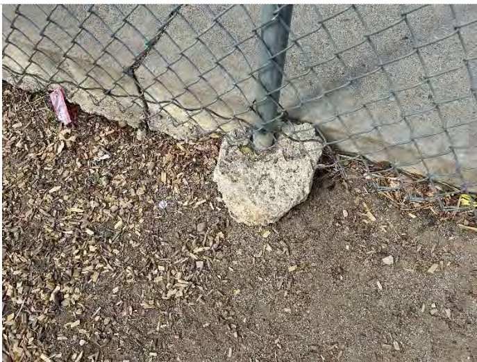
Concrete Fence Footings
