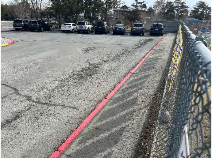
Red Paint on Concrete Curb
