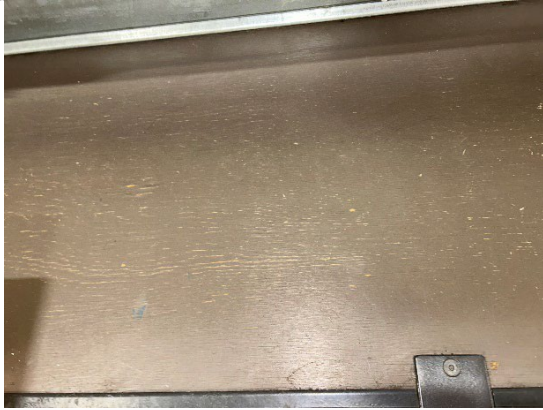
Brown Paint on Bleacher Foot Board
