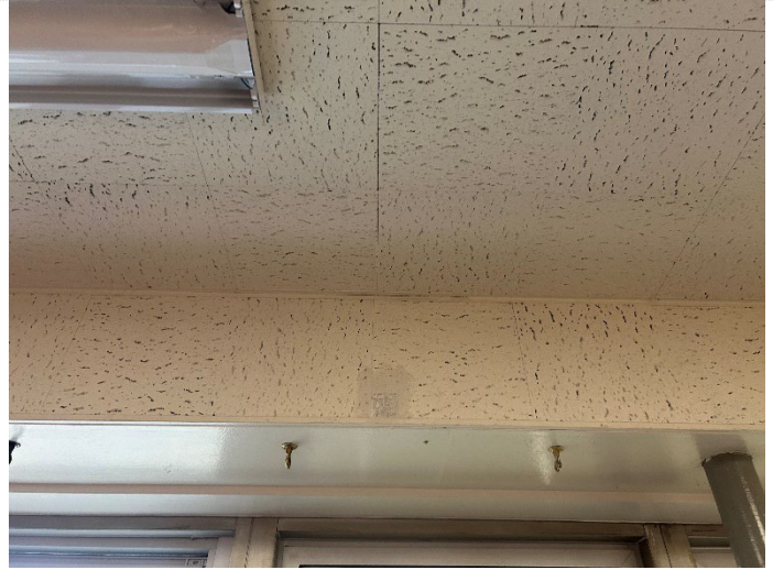
ACT – 12" Pinhole Fissure
