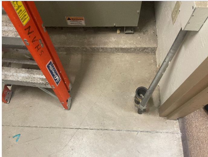
Concrete Grey Paint on Metal Electrical Box
