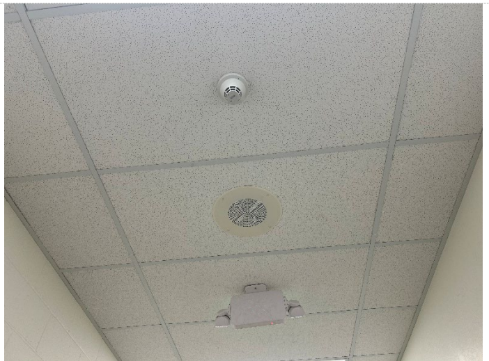
FCP – 2' x 4 Pinhole Fissure White Paint on FCP Ceiling
