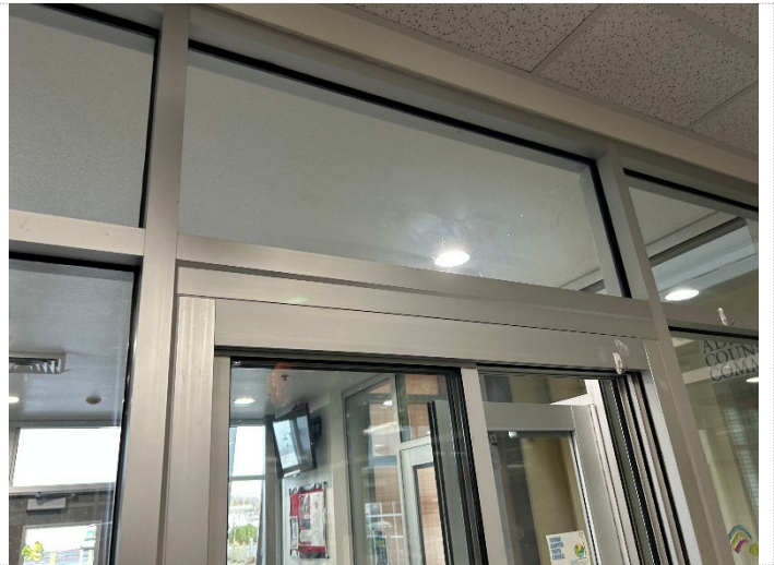
Silver Paint on Metal Window Frame
