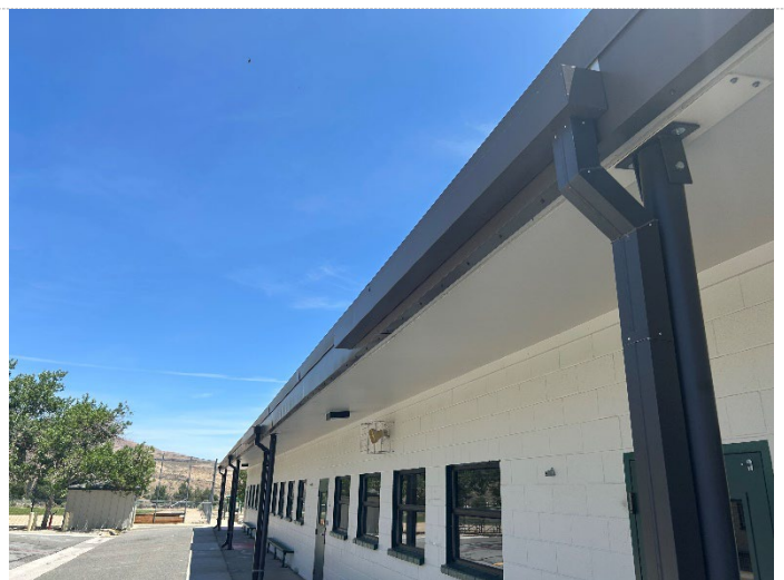
Brown Paint on Metal Flashing & Gutter
