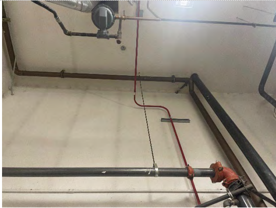
Black Paint on Metal Pipe
