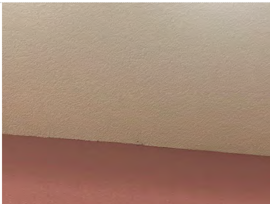
Maroon Paint on Drywall Wall
