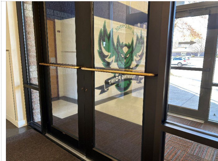
Brown paint on metal door
