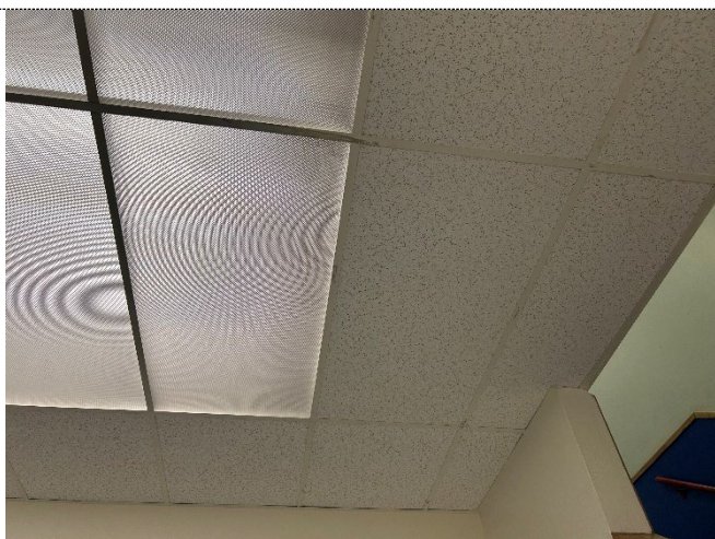
FCP – 2' x 4' Pinhole Fissure
