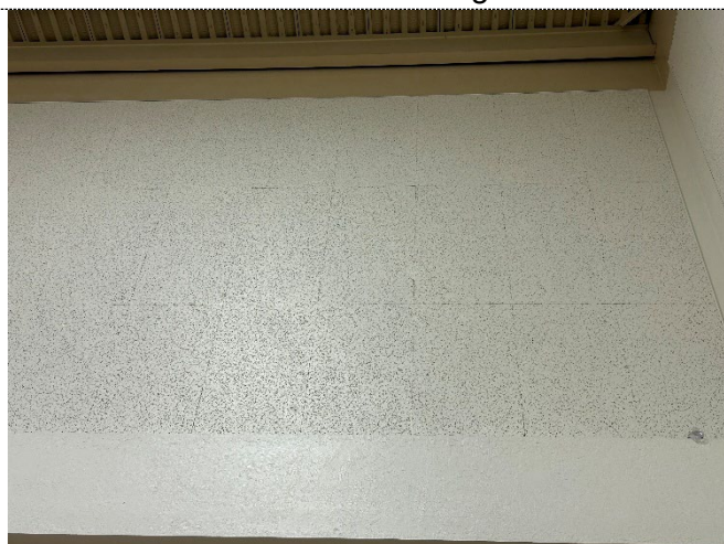
ACT & Glue – 2’ x 4’ Pinhole Fissure
