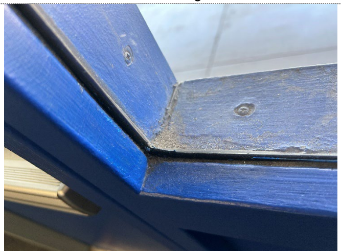
Window Frame Sealant
