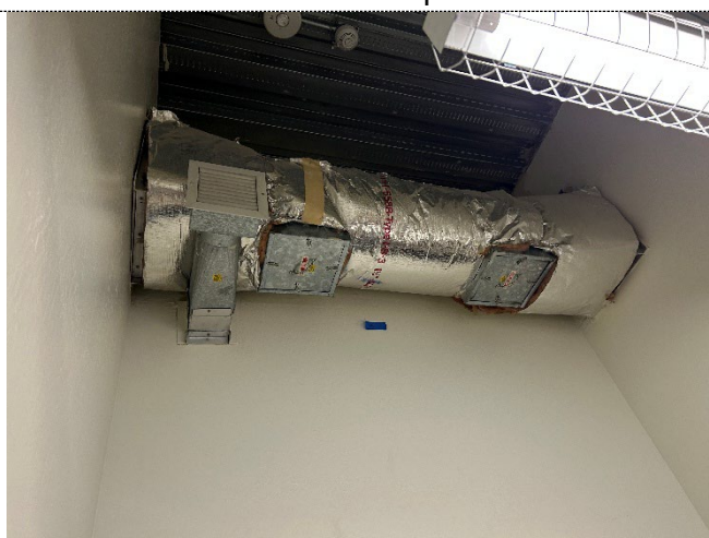
Fiberglass Duct Insulation
