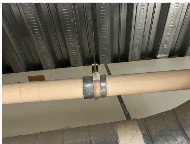
Pipe Hanger Insulation
