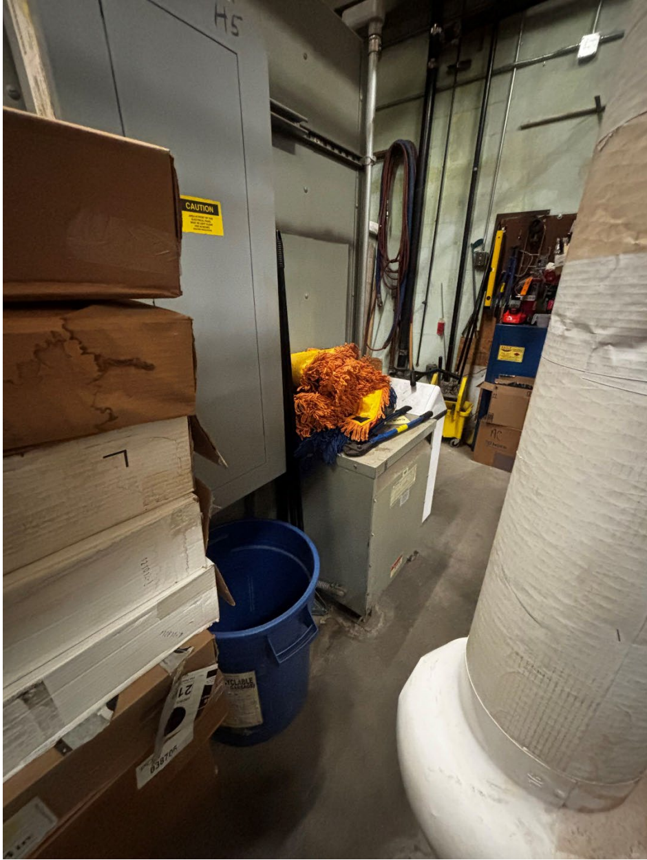
Access between heating boiler piping and building switchgear.
