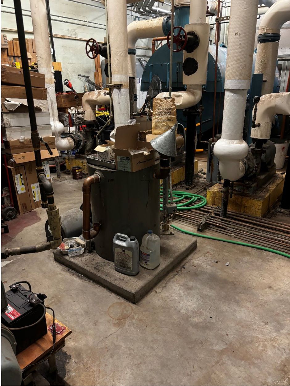
Glycol tank to be removed (view from backside.)
