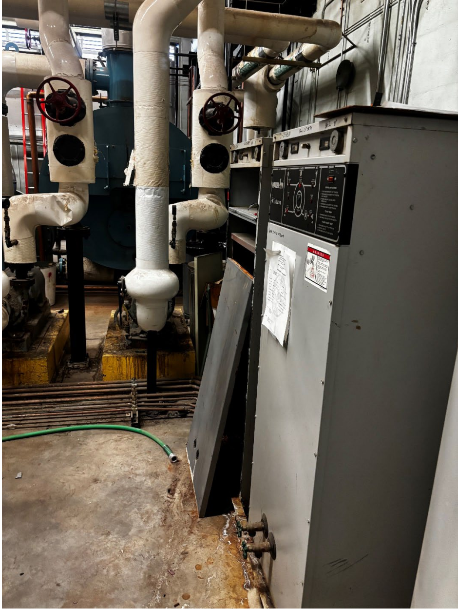
Front of existing domestic water boilers.
