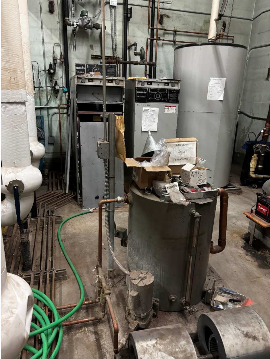
Glycol tank to be removed (Front view.)
