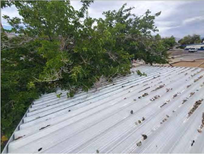
Trees Overhanging Roof Area
