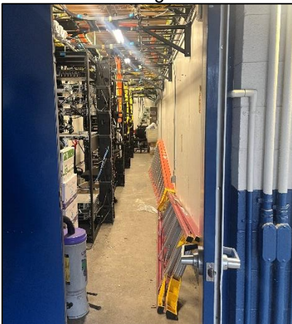
Building B server room
