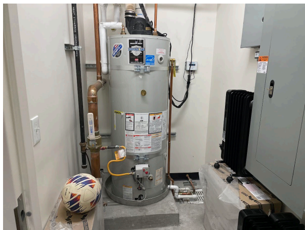
Newer Water Heater Servicing Counselor Offices
