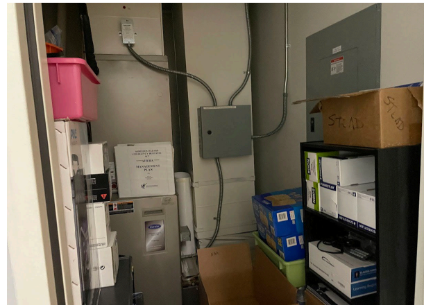
One of Several Electrical/Mechanical Rooms
