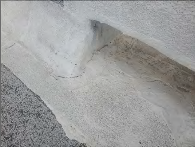
Base Flashing Split
